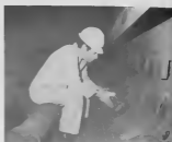
R. Amaya concentrating on condition observed in steam drum of boiler No. 7.
